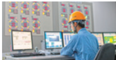
24-hour centralized control system
