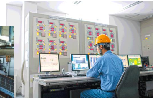
24 hour centralized control system
